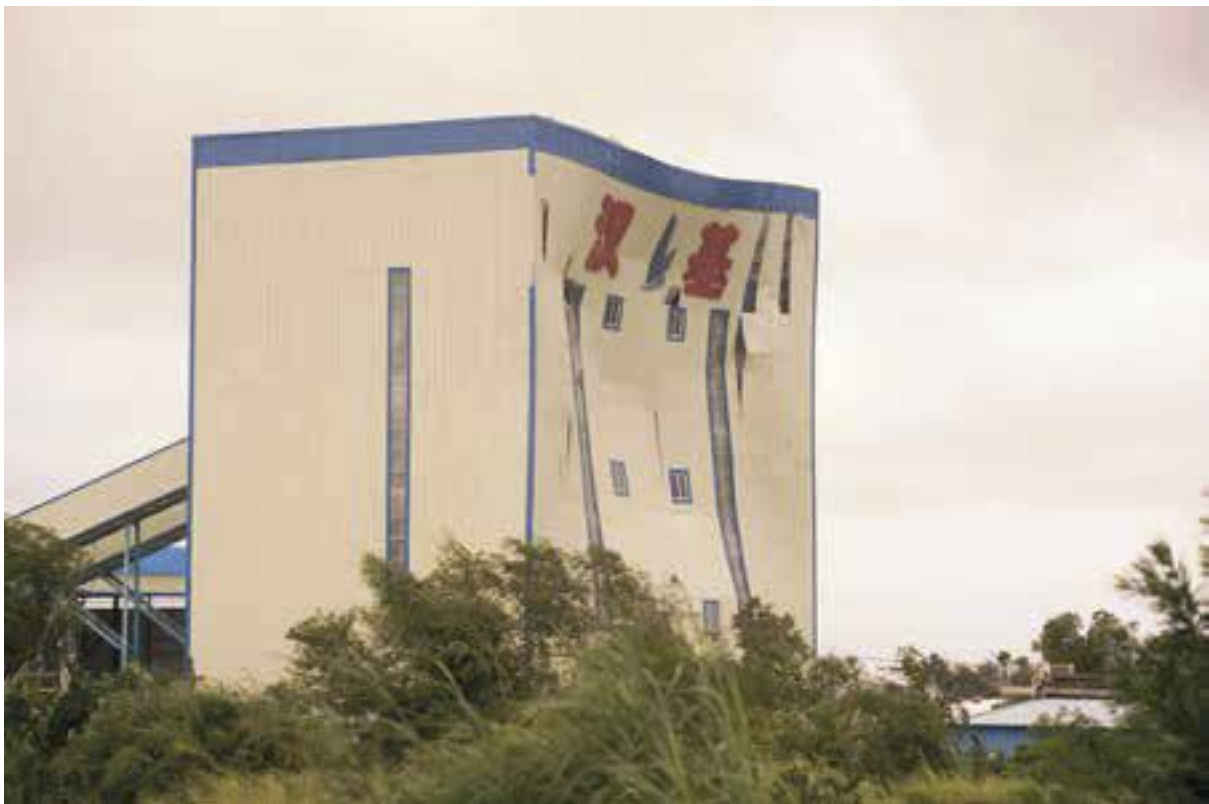
A damaged factory due to Typhoon Mangkhut in Zhuhai, Guangdong Province, China | Source - Getty Images
