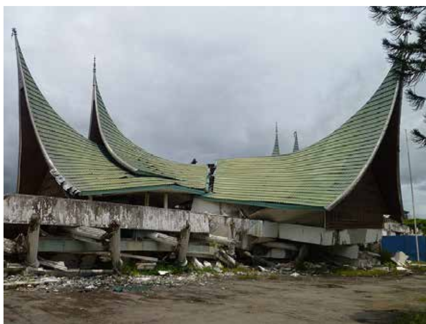
Damage from the Sep 30, 2009 Padang earthquake | Source: AusAID
