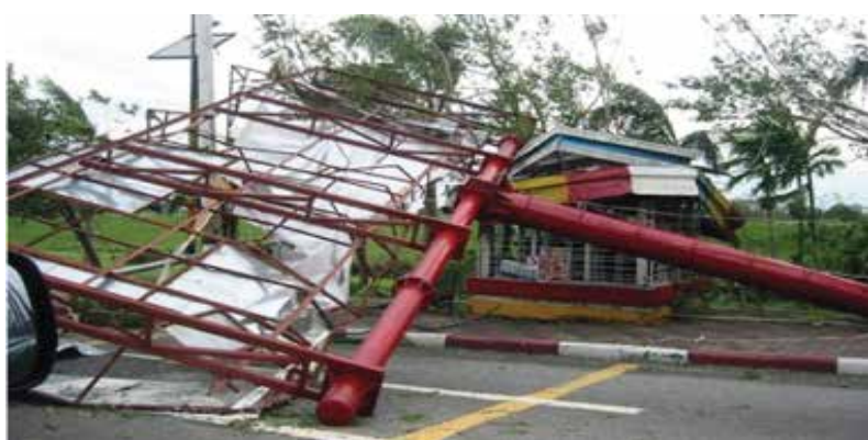
Damaged sign board during Cyclone Nargis 2008 Source: US Department of States
