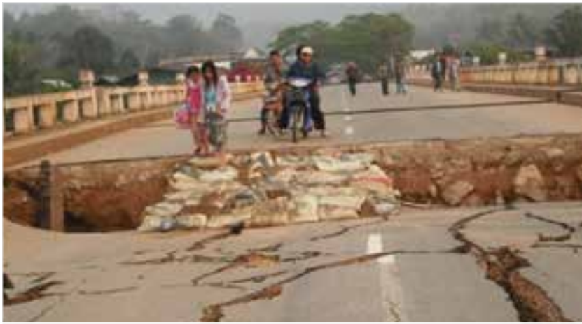
Damaged Road during March 24, 2011 earthquake
