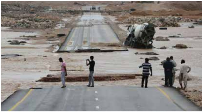
The Flood Tore Apart Whole Roadways during Cyclone Mekunu in May 2018 | Source: AP, abc.net.au
