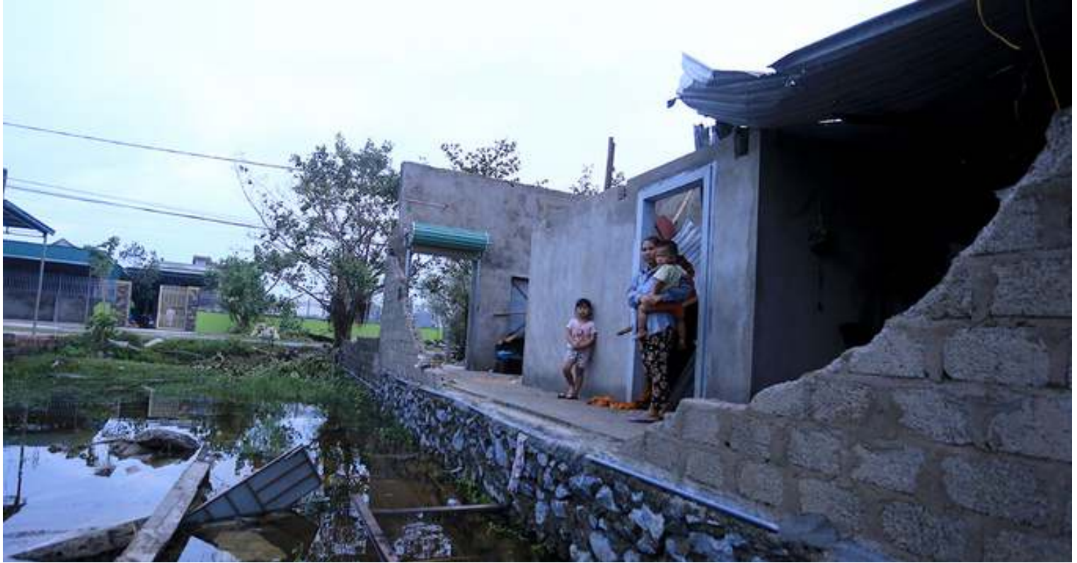
Damaged House During Typhoon Doksuri 2017 | Source: saigoneer.com
