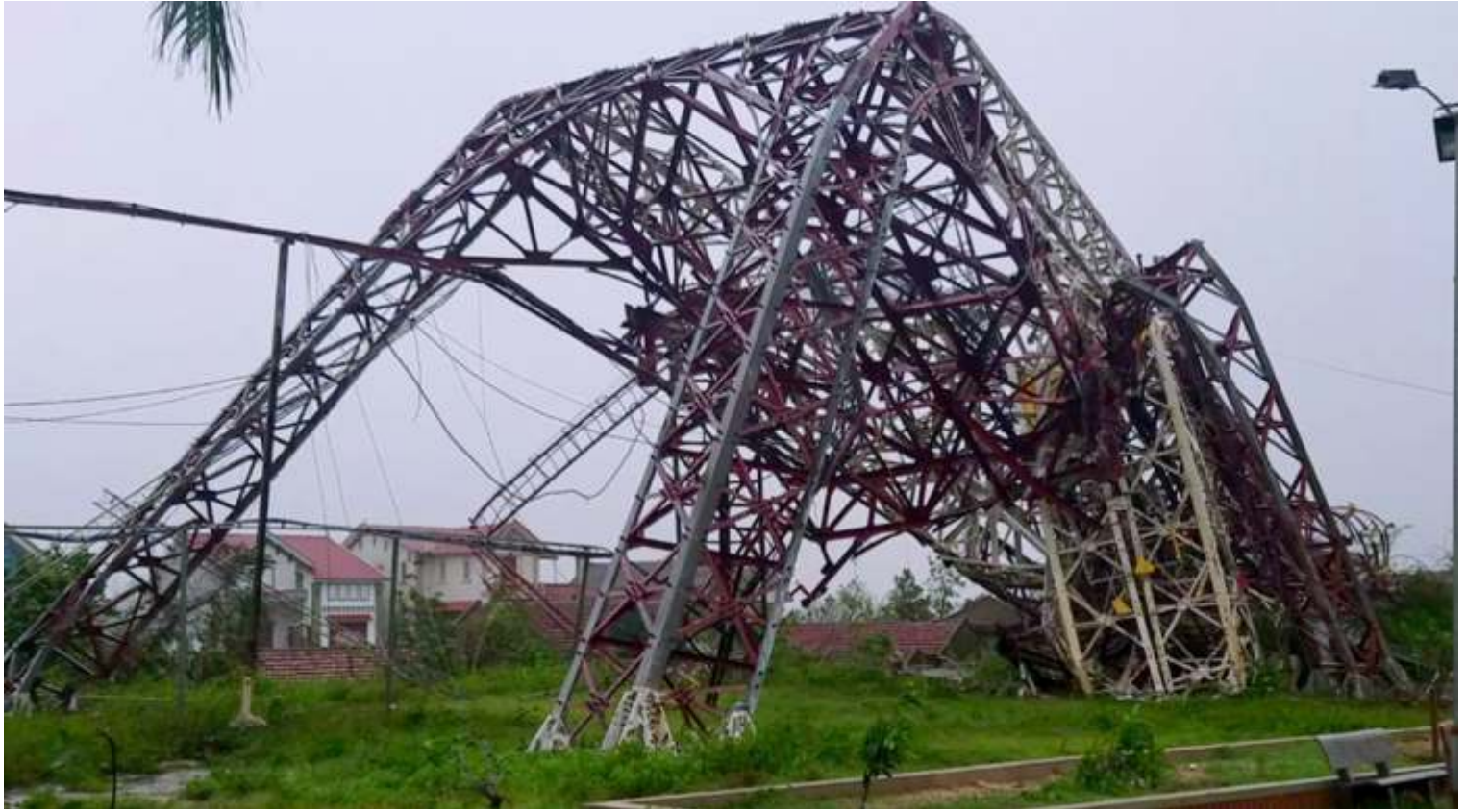
Damaged High Tension Pole During Typhoon Doksuri 2017 | Source: saigoneer.com
