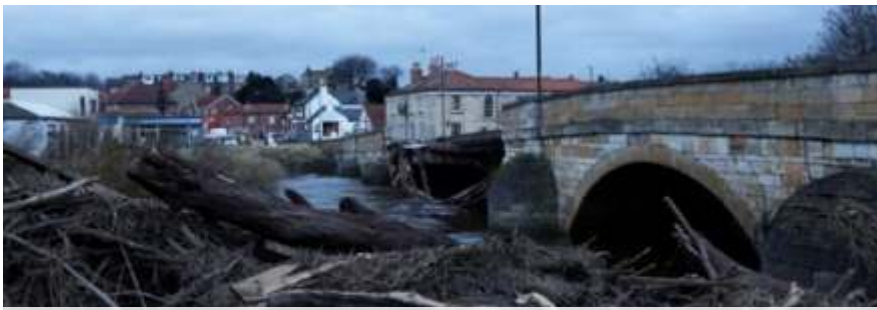
Collapsed bridge over the River Wharfe is seen in the market town of Tadcaster, North Yorkshire, Britain December 30, 2015. Source: Reuters/Craig Brough
